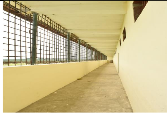
Block 1 after refurbishment works that addressed the cracks and enhanced security along the corridor and painting
